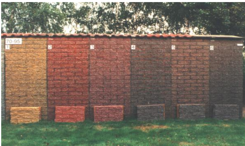
Photo 5: Concrete masonry blocks (un-weathered reference samples in foreground), Weathering commenced: 1970, Photo taken: 1995
